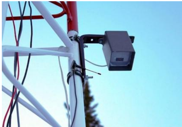
Figure 7. Receiver of data from a snow-temperature measuring rail.
