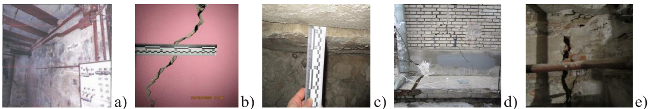
Fig. 1. Photo fixation examples of observed damage to the BTE object:
